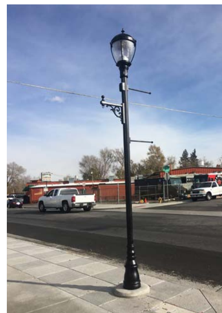
Newly installed pedestrian lighting with banner and planter arms
